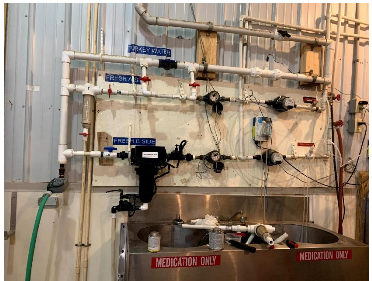
1" pipe, in-line livestock installation + drain
