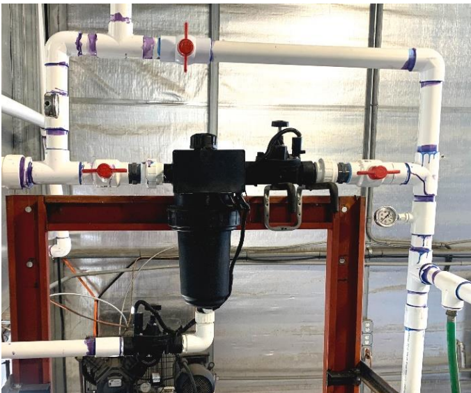
2" pipe, with bypass, nursery installation
